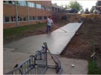
A wider sidewalk is poured outside lower level at the Middle School
