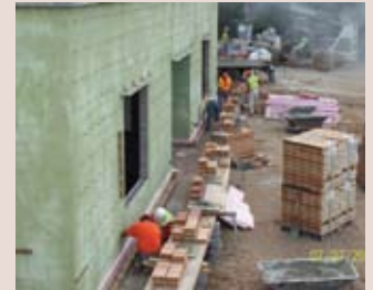
1st rows of exterior brick are laid at new Taylors Falls addition
